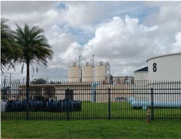
Lauderhill's water treatment plant will be upgraded with new treatment units, pumps and control software
