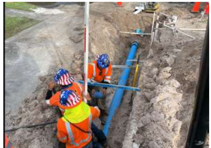
Replacement of water lines on Lime Hill Road and NW 82 Ave were completed during 2025
