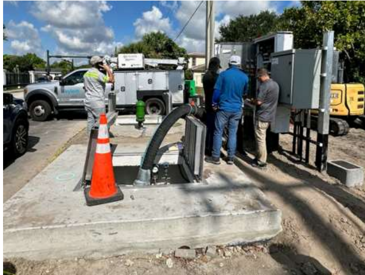
Lift station # 15 being tested prior to starting operations. Final phase is restoration of curbing and sidewalks.
