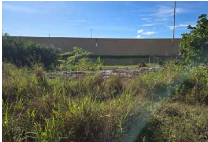
Preliminary clearing and grubbing work has started on the drainage improvements east of the Florida Turnpike
