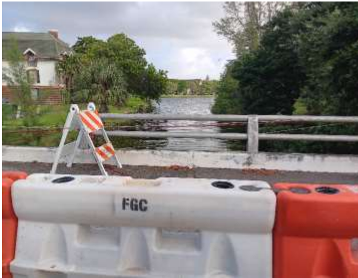
FG Construction completed bridge repair work in Inverrary to include two on Inverrary Blvd and one on Inverrary Drive
