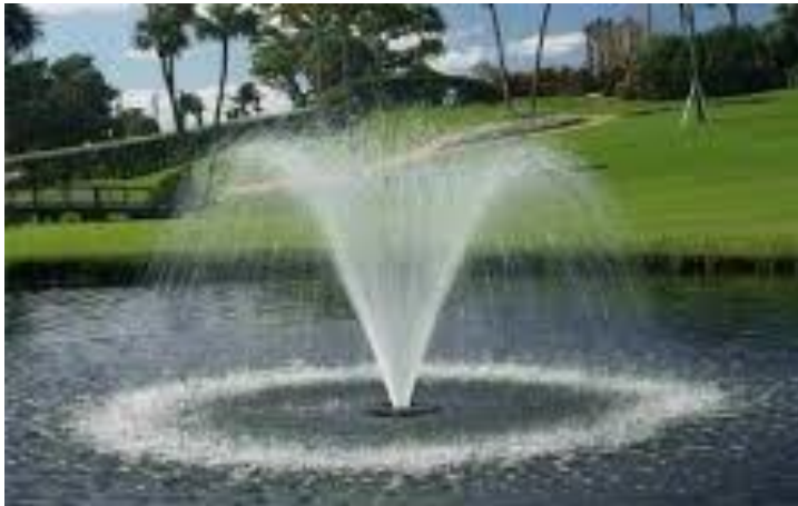
Park fountain pumps will be replaced as part of the project
